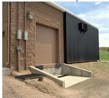
NREL Chemical Storage building, Golden, CO (Transpired solar collectors -2005) IAC Student Meeting
