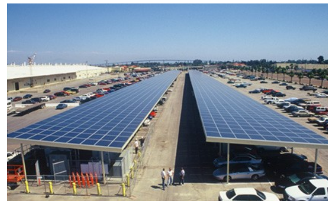
Naval Air Station, San Diego, CA (750 kW PV –2005)
