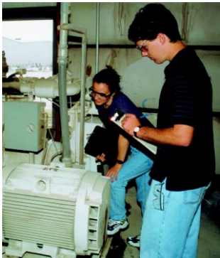
Engineering students, supervised by their professors, record their observations of a compressor operation at a recent IAC assessment.
