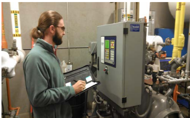
Michael Koch collecting data from an ammonia screw compressor at a local seafood processor.
